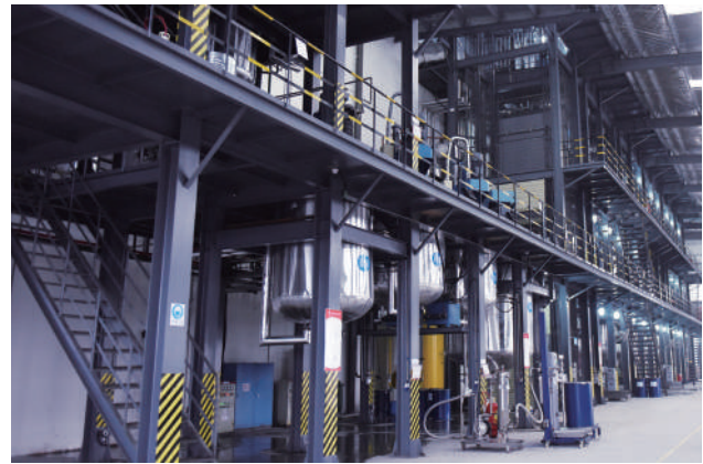
International leading polyurethane adhesive production line
